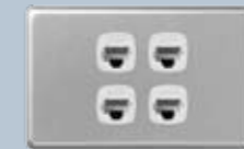
Telephone and computer outlets
